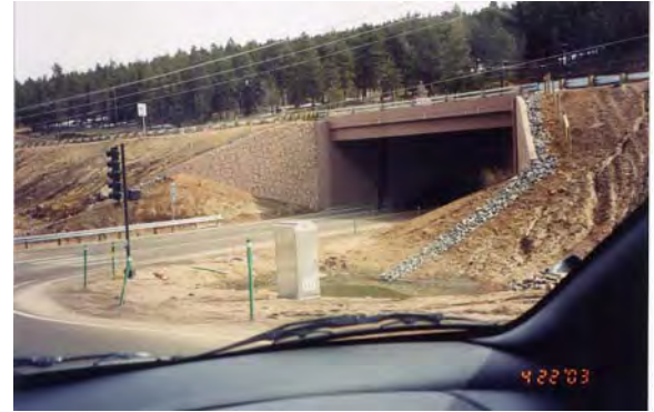
Grade-separated intersection with underpass at Conifer. Note vertical face abutments of the bridges placed near the edge of shoulder
